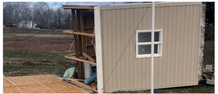
Picture 3: Wind Damaged Pool House
